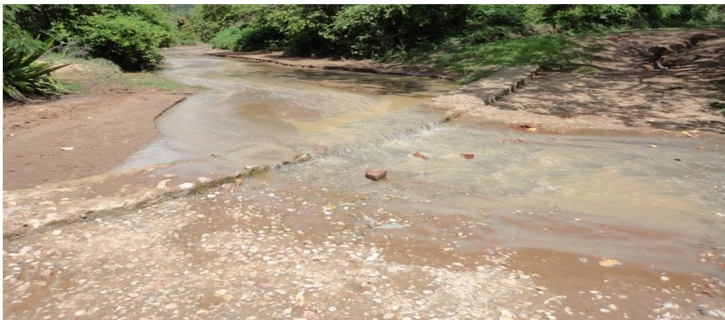
Plate 1: Sand dam at intersection of a road and river at Mutende, Kitui County, Kenya
